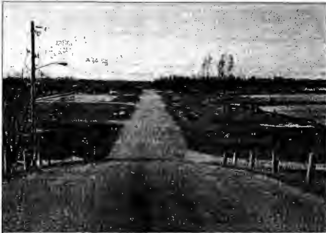
Southern section of Bayou Road and parking lot. See light brown areas that have been sawcut and filled with base material. Hot mix overlays and further repairs are still needed.
