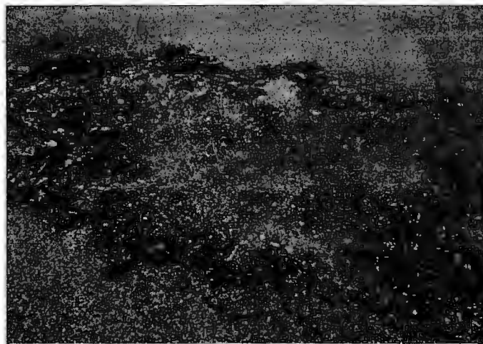
Sample depressions and base failure caused by debris trucks driving on roadway that had been saturated due to the tidal surge inundating the area.
