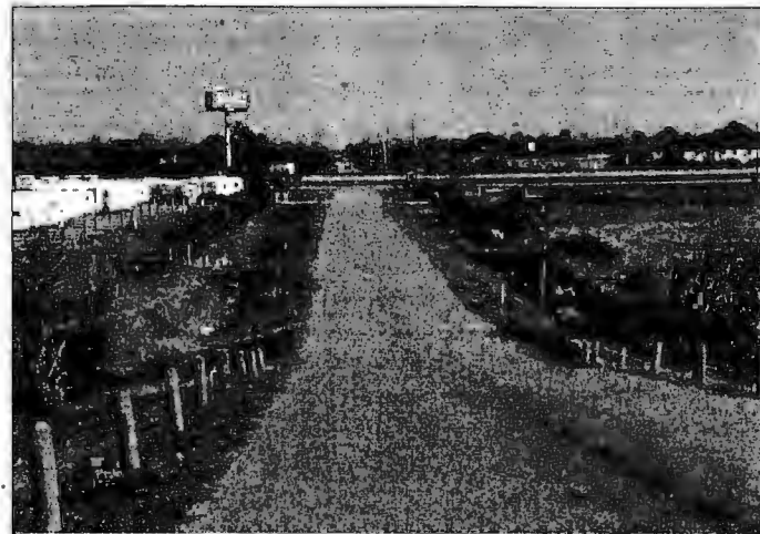
Northern section of Bayou Road. This section had not been inundated. Note the road did not become saturated and thus when heavy trucks used it, no failure of base was evident.
