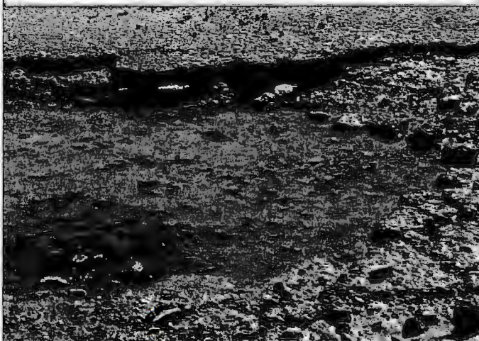
Eroded out and pavement failure due to subsidence of malleable and saturated base layers evident in close-up of pavement.
