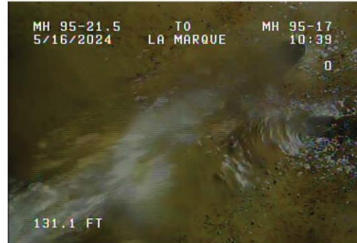
6, 00:06:33, 131.10ft Infiltration Gusher Barrel at 12 o'clock
