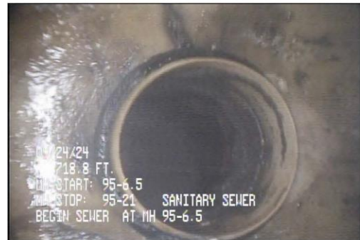
26, , 719.00ft Tap Rehabilitated Intruding at 12 o'clock, dia/height: 5inch, intruding: 1inch
