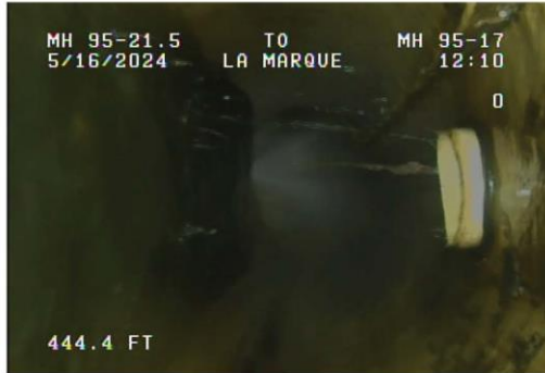
13, 00:19:58, 447.80ft Tap Factory Made Intruding at 12 o'clock, dia/height: 4inch, intruding: 1inch
