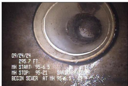
7, , 296.00ft Tap Rehabilitated Intruding at 12 o'clock, dia/height: 4inch, intruding: 1inch
