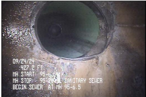
13, , 427.00ft Tap Rehabilitated Activity at 12 o'clock, dia/height: 4inch
