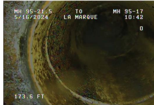
10, 00:08:46, 173.60ft Tap Factory Made Active at 12 o'clock, 4.000inch dim
