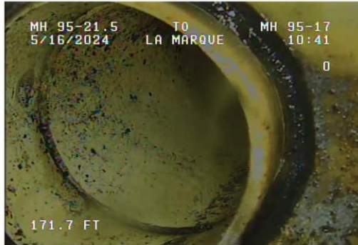
9, 00:08:18, 172.70ft Tap Factory Made Active at 12 o'clock, 4.000inch dim
