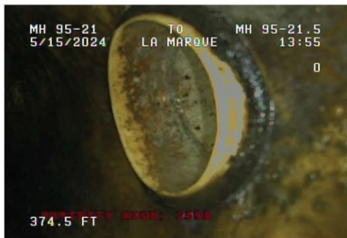
11, 00:12:24, 374.50ft Tap Factory Activity at 1 o'clock, dia/height: 4inch
