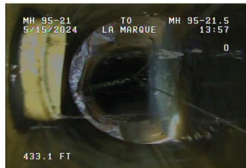
12, 00:14:34, 429.00ft Tap Factory Made Intruding at 12 o'clock, dia/height: 4inch, intruding: 2inch
