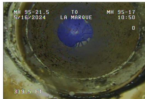
12, 00:16:44, 339.50ft Tap Factory Made Capped at 12 o'clock, 4.000inch dim
