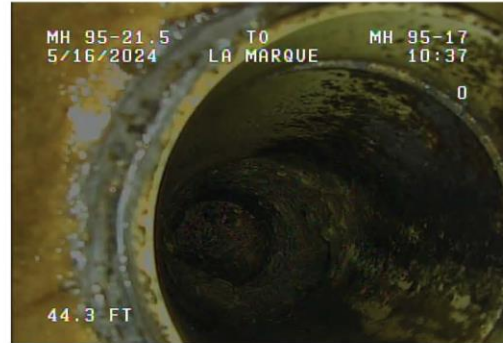
2, 00:03:56, 44.30ft Tap Factory Made Intruding at 12 o'clock, dia/height: 4inch, intruding: 1inch
