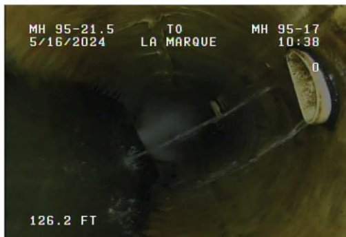
3, 00:05:48, 129.90ft Tap Factory Made Intruding at 12 o'clock, dia/height: 4inch, intruding: 1inch
