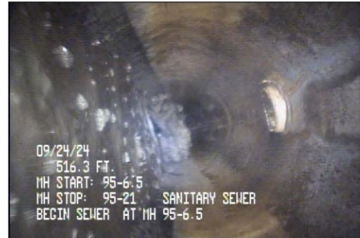
18, , 521.00ft Tap Rehabilitated Intruding at 12 o'clock, dia/height: 4inch, intruding: 1inch
