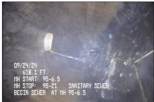
23, , 623.00ft Tap Rehabilitated Intruding at 11 o'clock, dia/height: 4inch, intruding: 1inch
