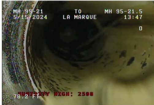
1, 00:03:28, 78.20ft Tap Factory Made Active at 12 o'clock, 4.000inch dim
