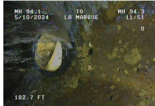
2, , 181.30ft Infiltration Gusher Connection at 12 o'clock
