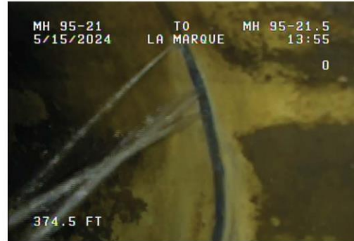
10, , 374.50ft Infiltration Gusher Joint from 11 o'clock to 4 o'clock, within 8 inch
