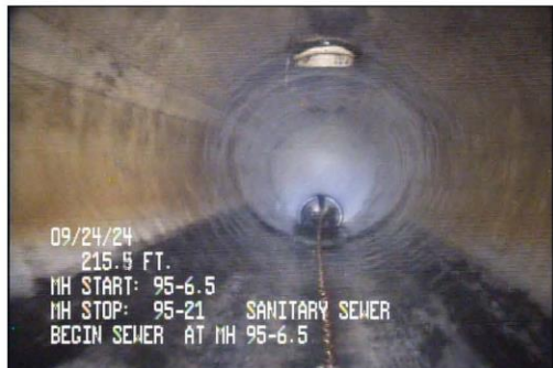
3, , 221.00ft Tap Rehabilitated Intruding at 12 o'clock, dia/height: 4inch, intruding: 1inch
