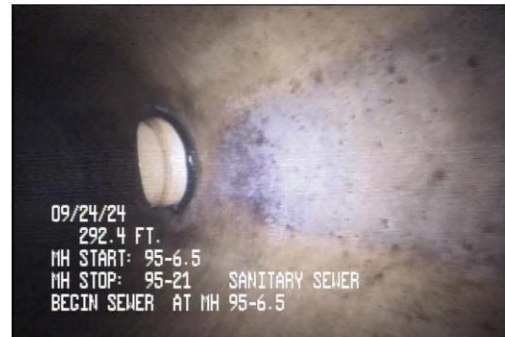
6, , 296.00ft Tap Rehabilitated Intruding at 12 o'clock, dia/height: 4inch, intruding: 1inch
