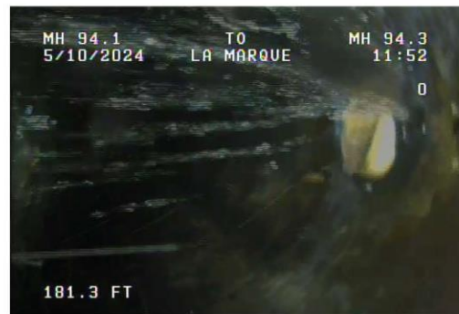
4, 00:05:06, 181.30ft Tap Factory Made Intruding at 12 o'clock, dia/height: 4inch, intruding: 1inch
