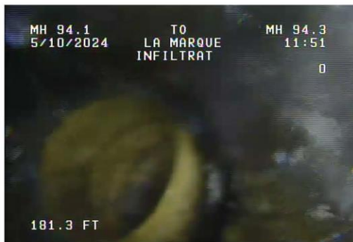
3, 00:05:06, 181.30ft Tap Factory Made Intruding at 12 o'clock, dia/height: 4inch, intruding: 1inch
