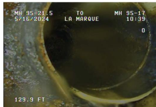
4, 00:05:48, 129.90ft Tap Factory Made Intruding at 12 o'clock, dia/height: 4inch, intruding: 1inch
