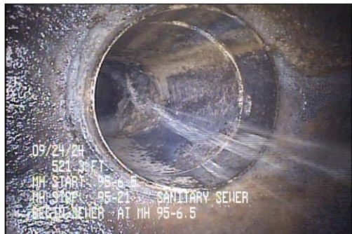
19, , 521.00ft Tap Rehabilitated Intruding at 12 o'clock, dia/height: 4inch, intruding: 1inch
