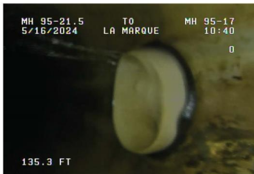
7, 00:07:04, 138.30ft Tap Factory Made Intruding at 12 o'clock, dia/height: 4inch, intruding: 1inch
