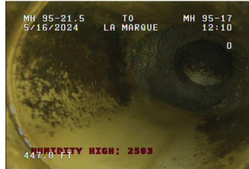
14, 00:19:58, 447.80ft Tap Factory Made Intruding at 12 o'clock, dia/height: 4inch, intruding: 1inch
