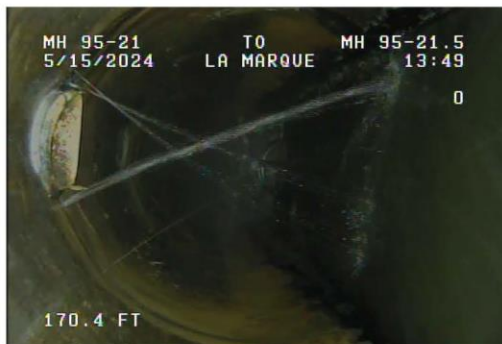
3, , 173.70ft Infiltration Gusher Connection at 12 o'clock
