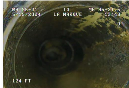
2, 00:04:40, 124.00ft Tap Factory Made Active at 12 o'clock, 4.000inch dim
