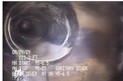
4, , 221.00ft Tap Rehabilitated Intruding at 12 o'clock, dia/height: 4inch, intruding: 1inch
