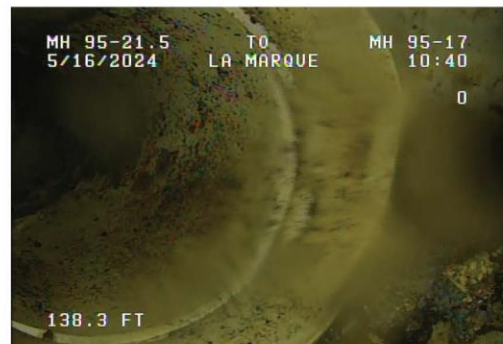
8, 00:07:04, 138.30ft Tap Factory Made Intruding at 12 o'clock, dia/height: 4inch, intruding: 1inch
