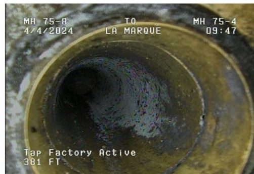
4, , 381.00ft Tap Factory Activity at 10 o'clock, dia/height: 4inch
