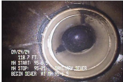
1, , 119.00ft Tap Rehabilitated Intruding at 12 o'clock, dia/height: 4inch, intruding: 1inch
