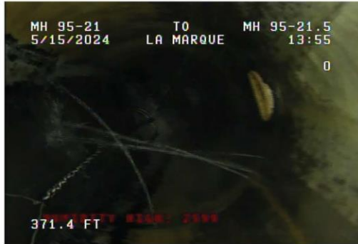
9, , 374.50ft Infiltration Gusher Joint from 11 o'clock to 4 o'clock, within 8 inch
