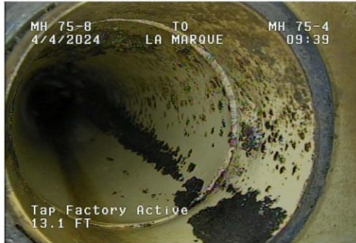
1, , 13.10ft Tap Factory Activity at 12 o'clock, dia/height: 4inch
