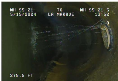
7, , 279.20ft Infiltration Gusher Connection at 12 o'clock
