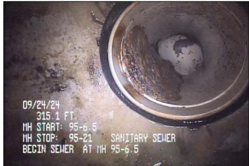
9, , 315.00ft Tap Rehabilitated Intruding at 12 o'clock, dia/height: 4inch, intruding: 1inch
