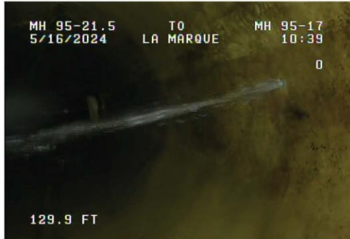
5, 00:06:33, 131.10ft Infiltration Gusher Barrel at 12 o'clock
