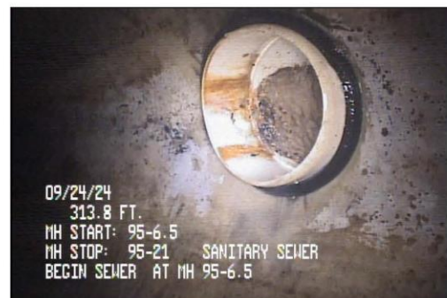
8, , 315.00ft Tap Rehabilitated Intruding at 12 o'clock, dia/height: 4inch, intruding: 1inch
