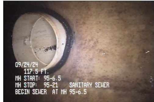
2, , 119.00ft Tap Rehabilitated Intruding at 12 o'clock, dia/height: 4inch, intruding: 1inch
