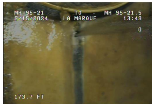
4, , 173.70ft Infiltration Gusher Connection at 12 o'clock
