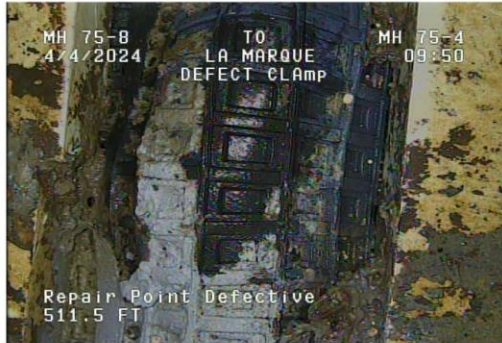
5, 511.50ft Point Repair Other Defective / CLAMP
