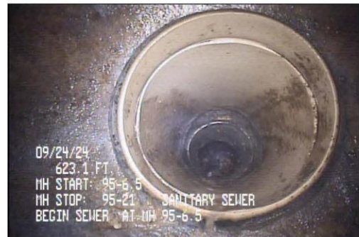
24, , 623.00ft Tap Rehabilitated Intruding at 11 o'clock, dia/height: 4inch, intruding: 1inch
