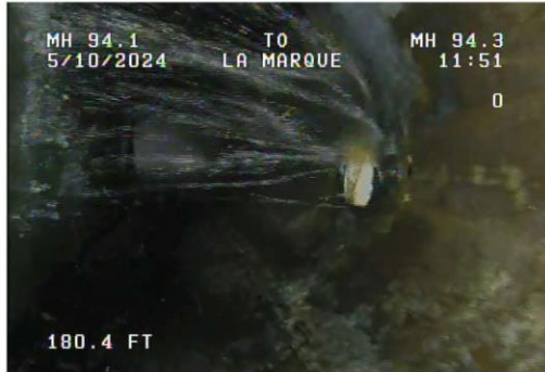
1, , 181.30ft Infiltration Gusher Connection at 12 o'clock
