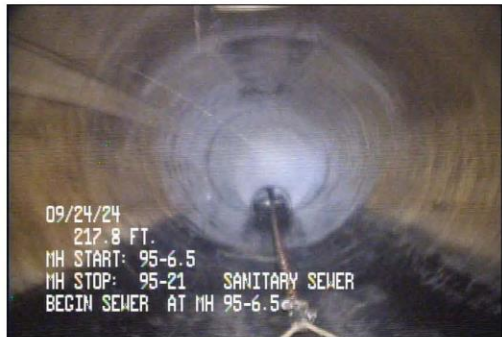
5, , 222.00ft Infiltration Gusher Barrel from 10 o'clock to 11 o'clock
