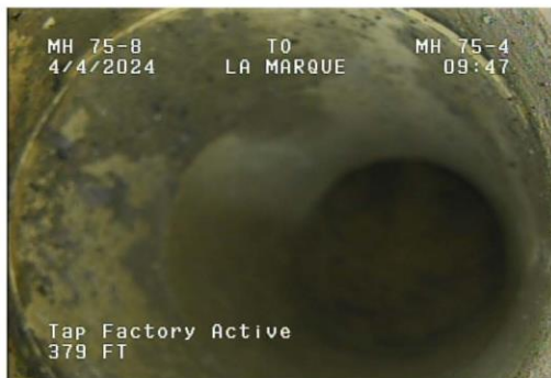
3, , 379.00ft Tap Factory Activity at 2 o'clock, dia/height: 4inch
