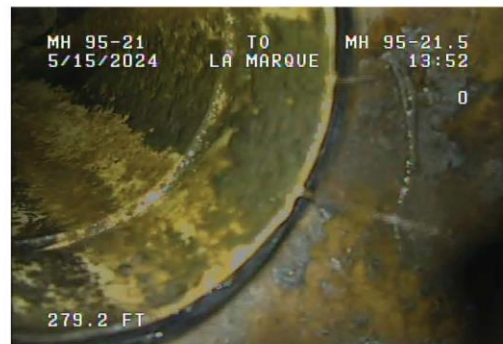
8, 00:09:11, 279.20ft Tap Factory Activity at 12 o'clock, dia/height: 4inch
