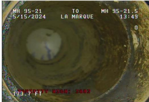
5, 00:06:06, 173.70ft Tap Factory Activity at 12 o'clock, dia/height: 4inch
