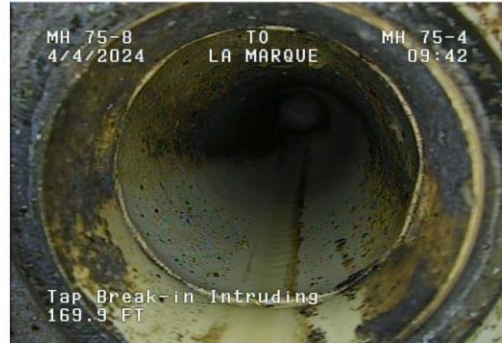
2, , 169.90ft Tap Factory Made Intruding at 10 o'clock, dia/height: 4inch, intruding: 2inch
