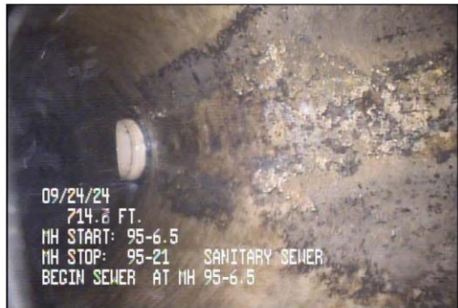
25, , 719.00ft Tap Rehabilitated Intruding at 12 o'clock, dia/height: 5inch, intruding: 1inch
