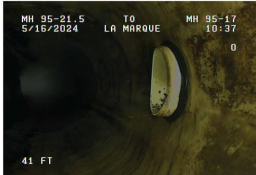
1, 00:03:56, 44.30ft Tap Factory Made Intruding at 12 o'clock, dia/height: 4inch, intruding: 1inch
